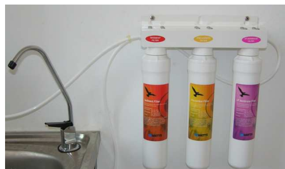
Triple system installed in a restaurant in Singapore
